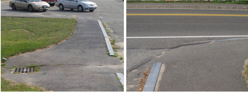
Problems with placement of drainage & cross slope issues and does not comply with ADA curbcut guidelines.
