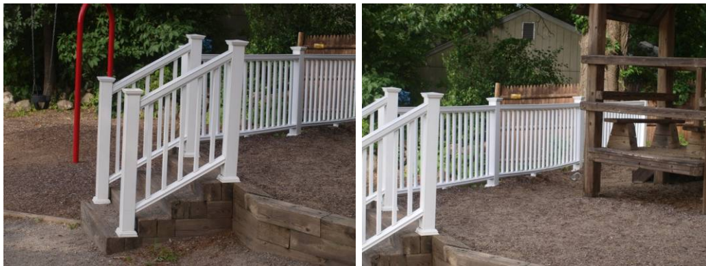
New stair railings were recently installed and do not meet ADA standards.
