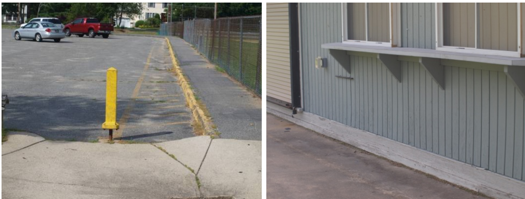
Bollard restricts access from parking area, concession stand shelf is too high for wheelchair service.
