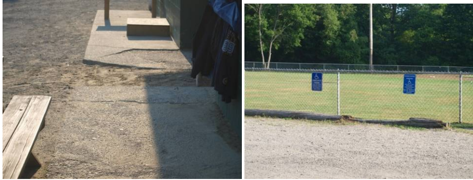
Broken sidewalk at concession stand and designated parking could be improved (see example at Martins Pond).
