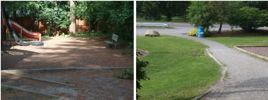
Wood chip and stepped playground surface inhibits access and ramp surface could be improved and signed.
