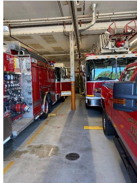
Open Doors Conflict with Structure
